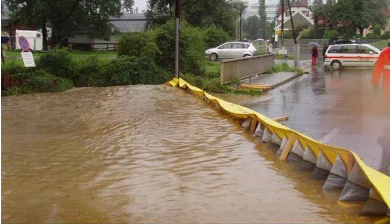
Figure 3-3: Temporary Flood Barrier – Rising Flood Water
