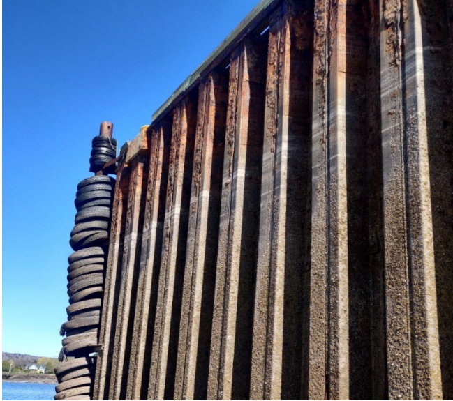
Figure 5 – Three Patches Near the High Water Mark on West Side of the Wharf in Good Condition
