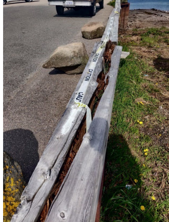
Figure 12 - Timber Curbs on East Side of Wharf Rotten
