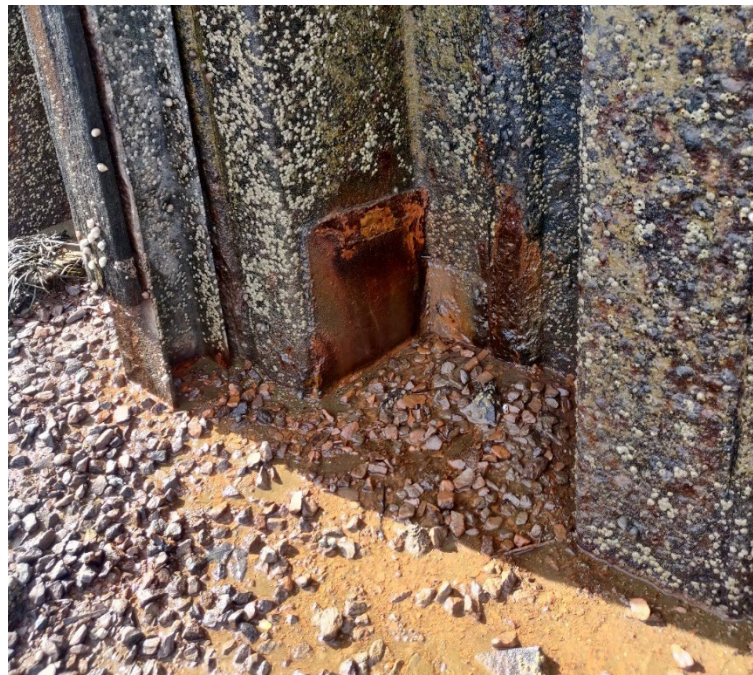
Figure 7 – Patch on East Side of Wharf Near the Bottom
