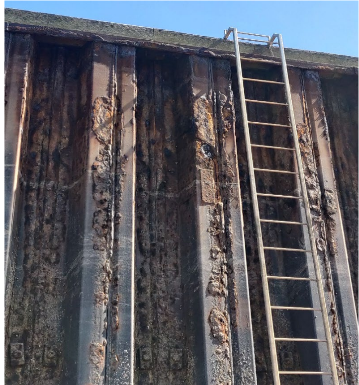
Figure 9 - New Portable Aluminum Ladder Installed in 2023
