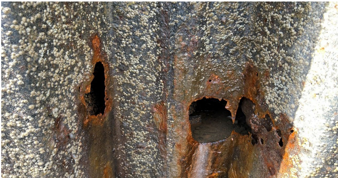
Sheet Pile on Lower East Side Nearly Rusted Through (requires urgent patch).
