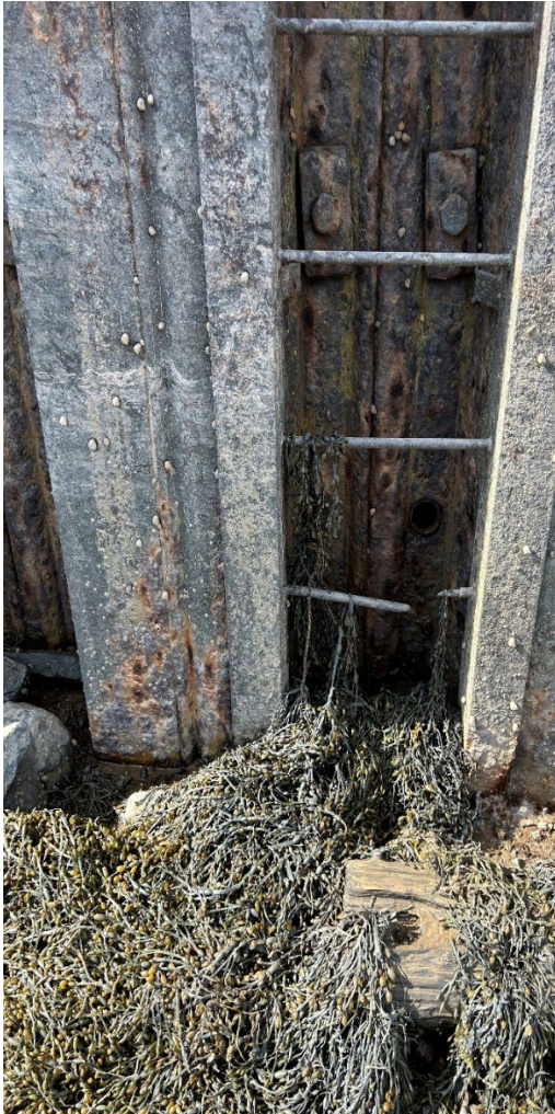
Figure 8 - Example of Damaged/Broken Ladder
