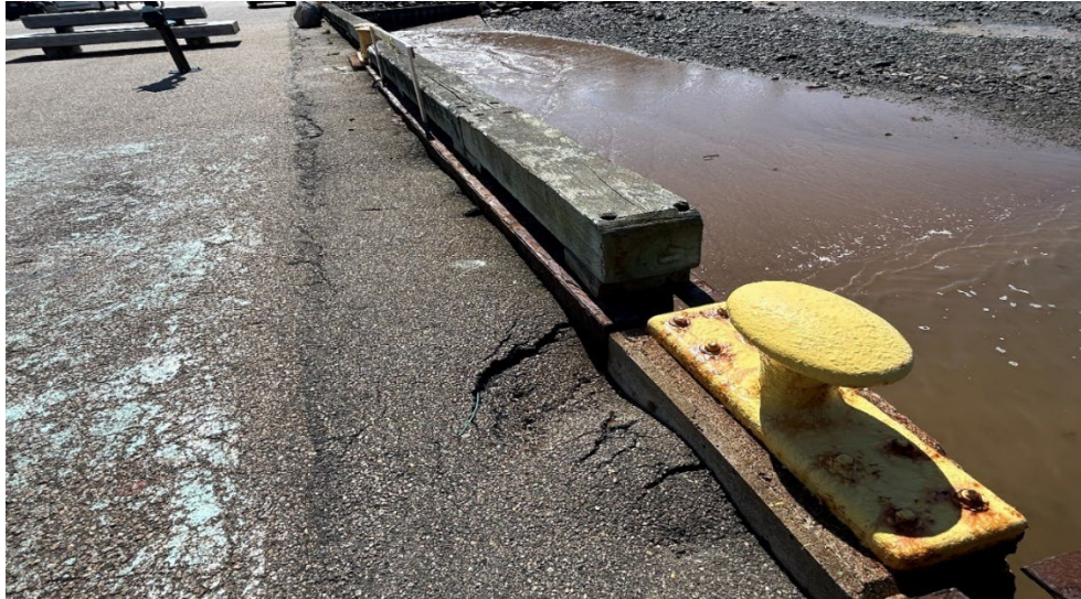
Figure 15 –Settling Along Sides of Asphalt Deck
