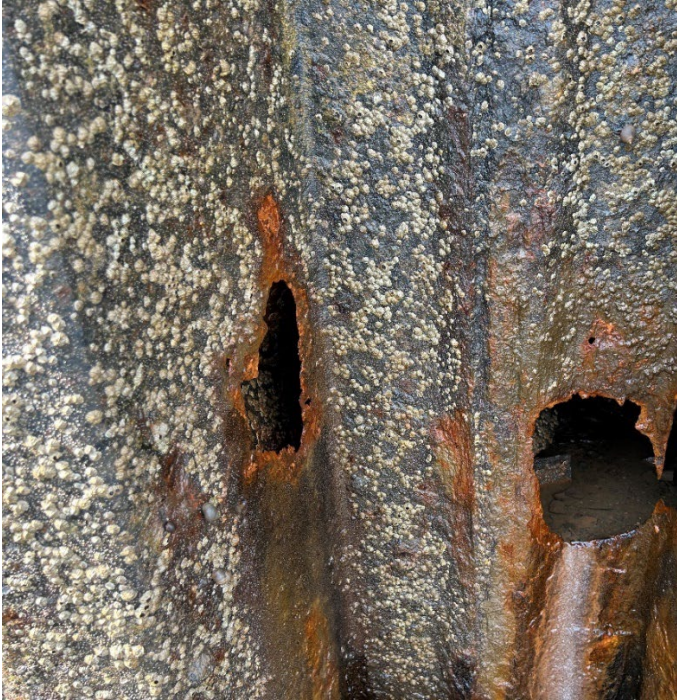
Figure 3 – Rust Deterioration on Lower East Side of Wharf
