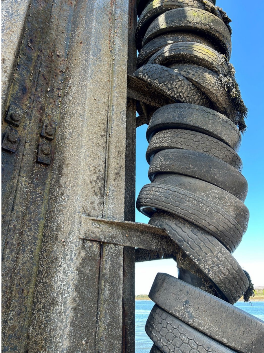
Tire Corner Fenders on North End of Wharf Still Intact
