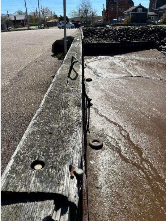
Figure 11 - Timber Curb with Fallen Tires
