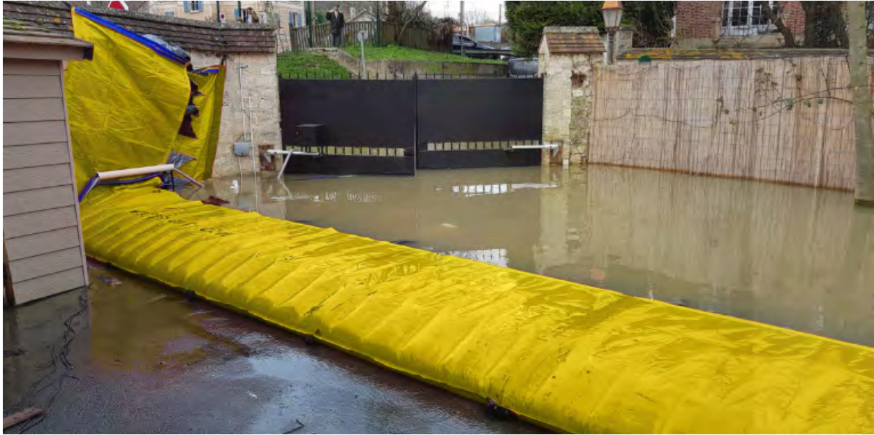
Figure 3-4: Flood Barrier in Place
