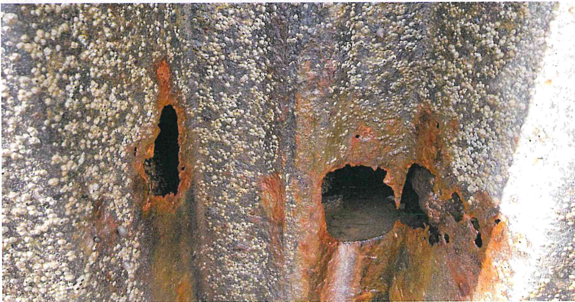
Sheet Pile on Lower East Side Nearly Rusted Through (requires urgent patch).
