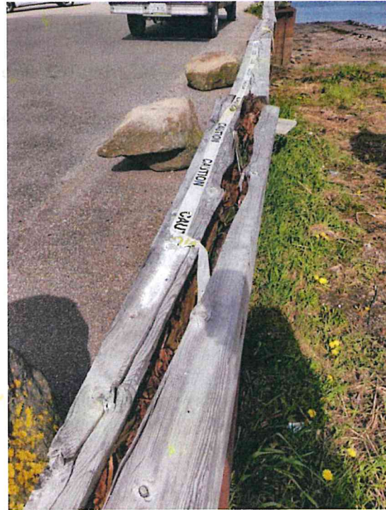
Figure 12 - Timber Curbs on East Side of Wharf Rotten
