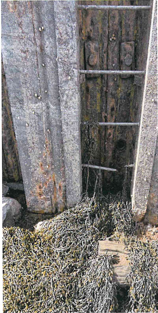
Figure 8 - Example of Damaged/Broken Ladder
