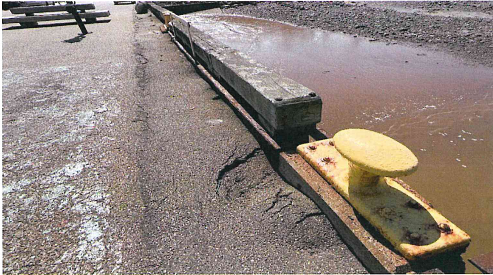
Figure 15 –Settling Along Sides of Asphalt Deck
