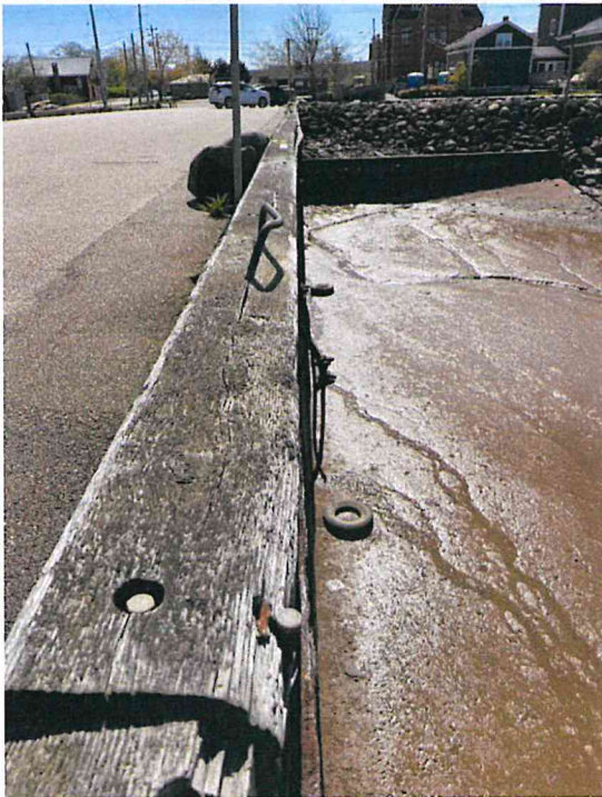
Figure 11 - Timber Curb with Fallen Tires
