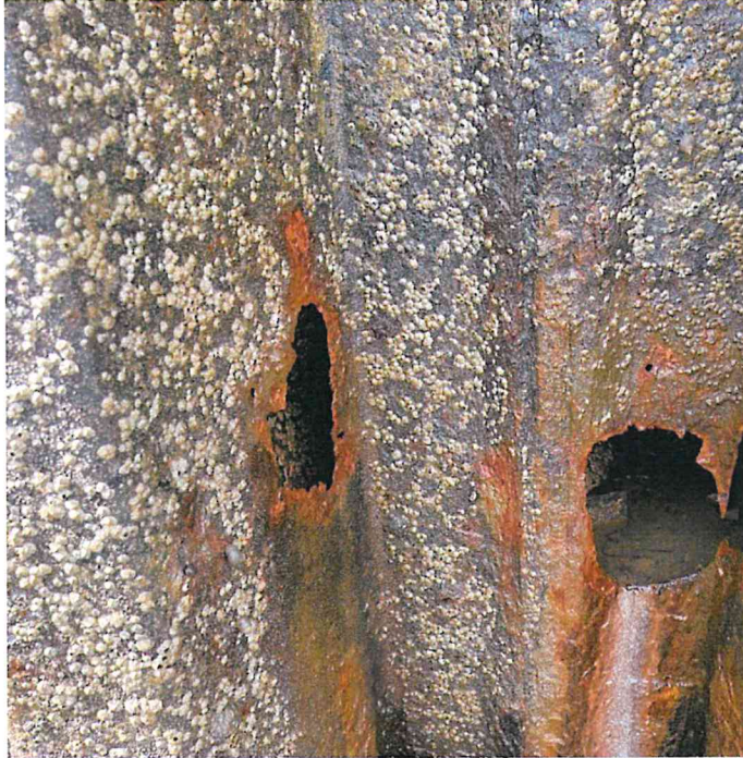
Figure 3 – Rust Deterioration on Lower East Side of Wharf
