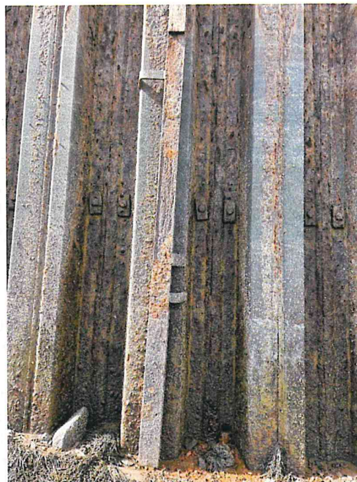
Figure 13 - Wooden Fenders on Side of Wharf Missing
