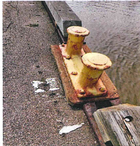
Figure 10 - Steel Bollards Anchored in Concrete
