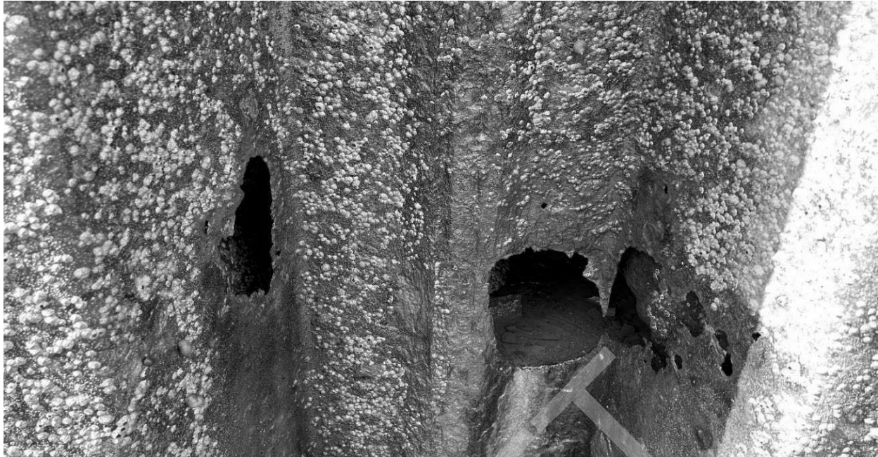
Sheet Pile on Lower East Side Nearly Rust Through (2024).
