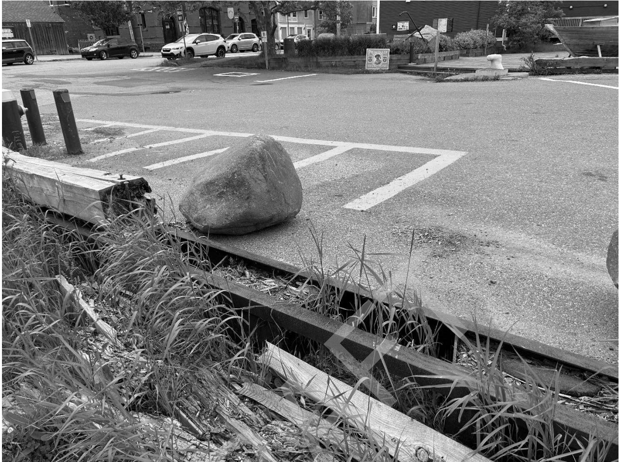
Wooden curb rotted away on east side of inner Wharf and large rocks place to keep cars from driving off
