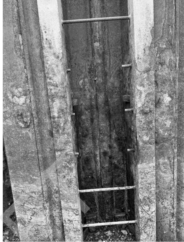
Figure 9 – Ladder on East Side with rungs removed.
