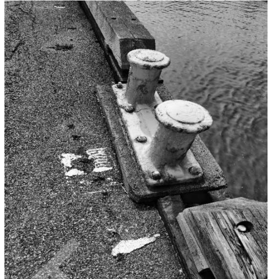
Figure 11 - Steel Bollards Anchored in Concrete
