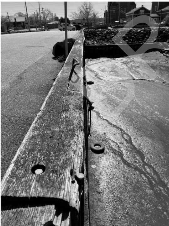
Figure 12 - Timber Curb with Fallen Tires
