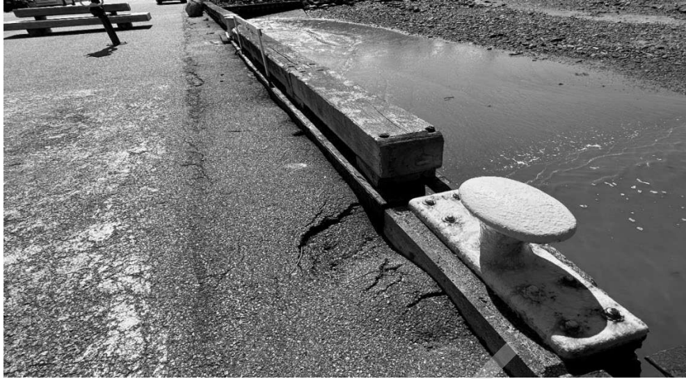
Figure 16 –Settling Along Sides of Asphalt Deck
