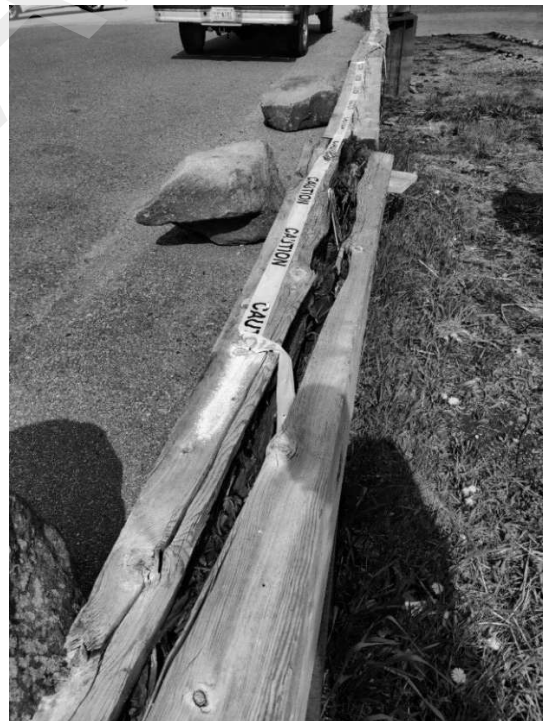
Figure 13 - Rotten Timber Curbs on East Side of Wharf
