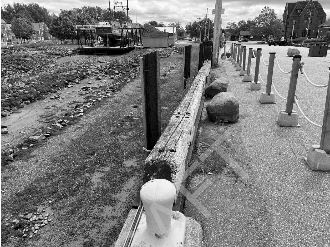
East side of outer wharf fenced off closing use of floating dock facility and keeping people away from the side.
