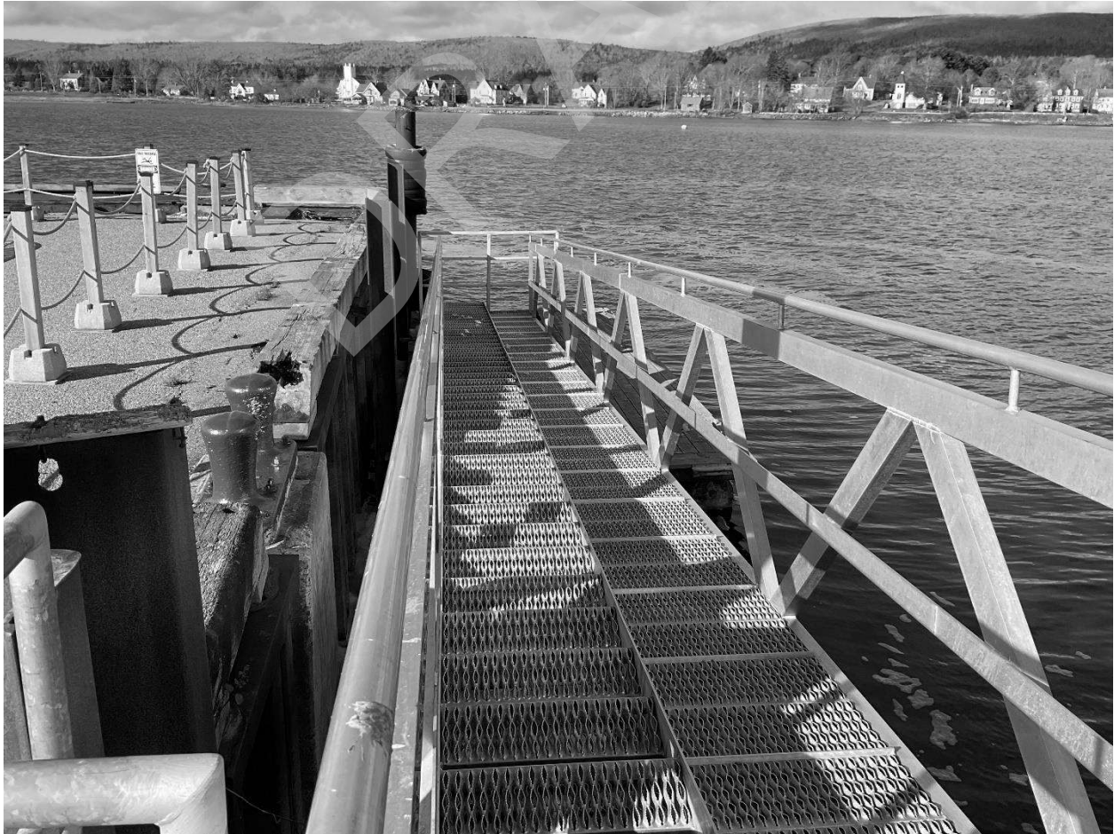
Floating Dock at High Tide
