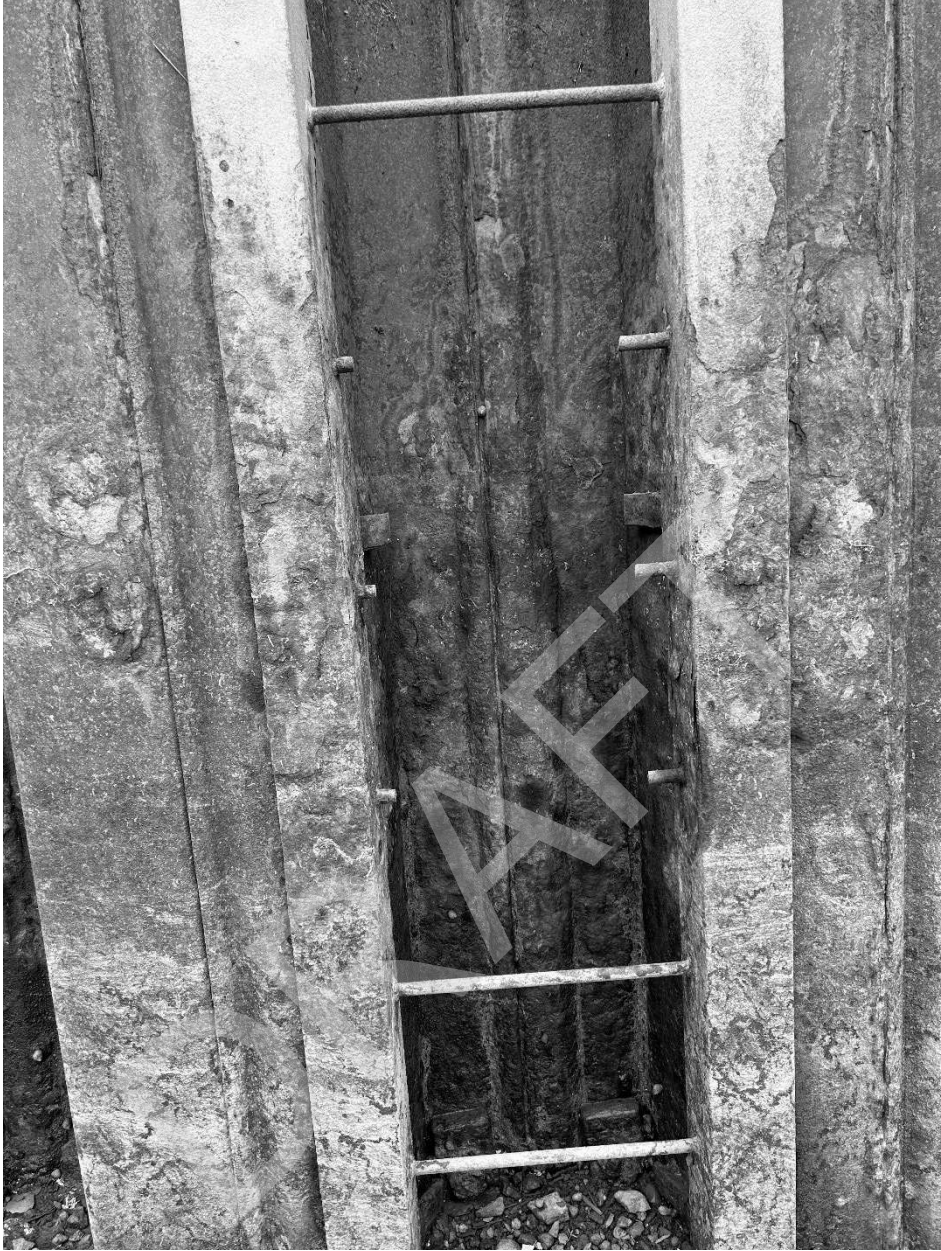
Steps cut out of ladder to discourage people climbing on them
