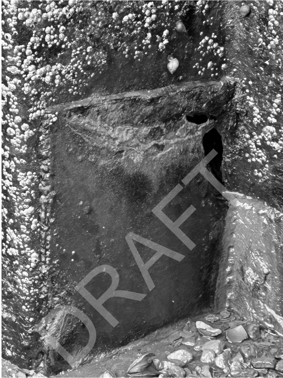
Patch on East side of wharf from a couple of years ago rusting through
