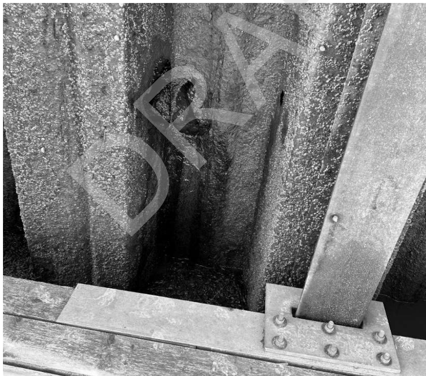
Figure 5 - Sheet Pile Deterioration at Drainage System Level, East Side of Wharf Near North End 2024
